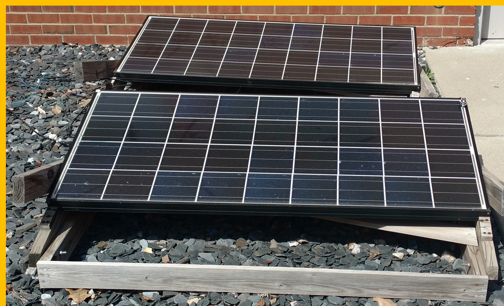
Solar panels located in the courtyard of Coover Hall
